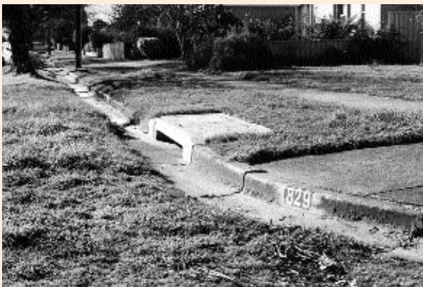
Dry weather side-entry pit
