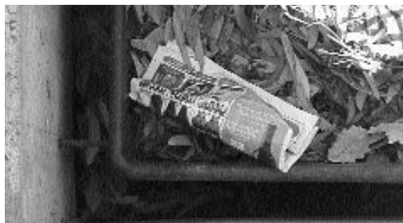
A litter basket placed inside a Side Entry Pit ® .
